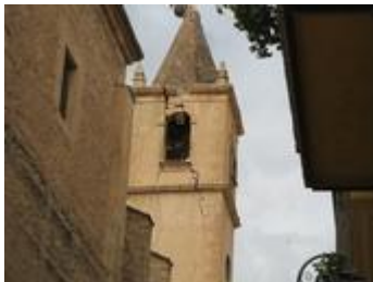
Earthquake in Lorca, Spain, 11 May 2011.
