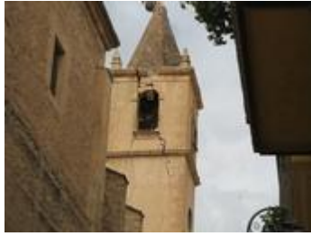
Earthquake in Lorca, Spain, 11 May 2011.
